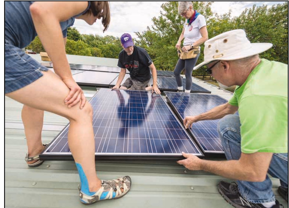
Volunteers from the Flint Hills Renewable Energy Co-op and the Salina community help with the placement of solar electric panels on the Research Building roof.
