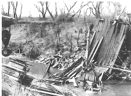
The demolished bridge, with the truck and backhoe that brought it down.
