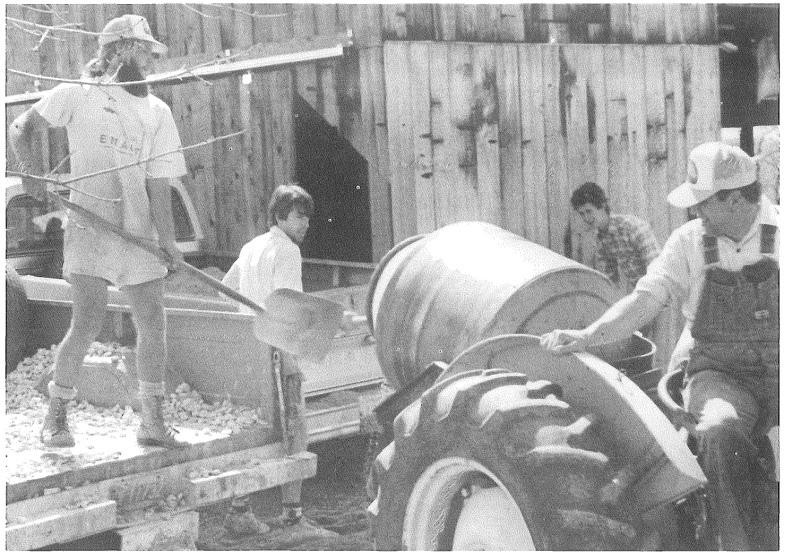
Mark S., Patrick B., Dennis R. and Wes J. mix concrete for east wall of new shop in red barn which Rob F. built. Doors on new barn in background were built by interns in February and March.
